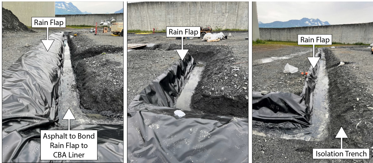
Figure 3. Photographs of installed rain flap (from WSP 2024a).
